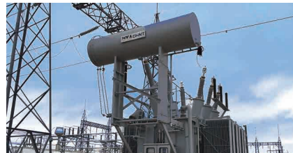
230kV 200MVA Autotransformer USA
