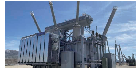
525kV 525MVA Autotransformer USA
