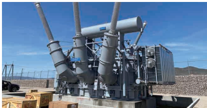
161kV 15MVA Reactor - Hydro QC Canada
