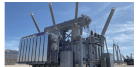
525kV 525MVA Autotransformer USA
