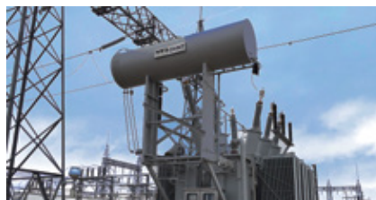
230kV 200MVA Autotransformer USA
