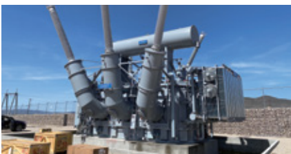
161kV 15MVar Reactor - Hydro QC Canada
